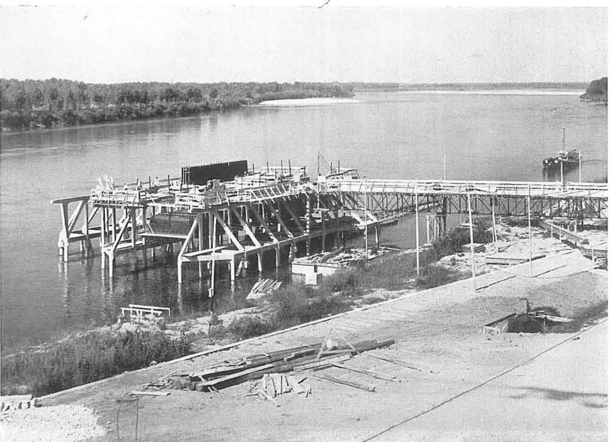
Dam - Deck on the right bank for construction of floating caissons - November 1958
