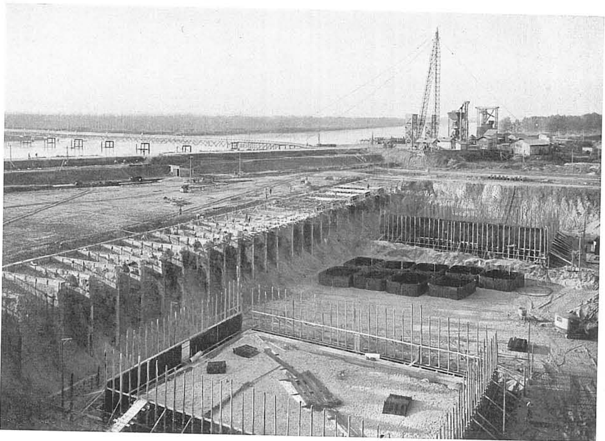
Powerhouse - Construction of the two pneumatic caissons for units I and IV (El. 28,00). On the left, supporting buttresses of the perimetral diaphragm, riverside wall - November 1958
