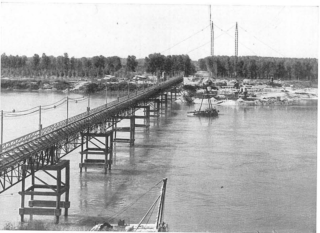
Dam - Temporary service footbridge and construction of piers on the left bank - September 1958
